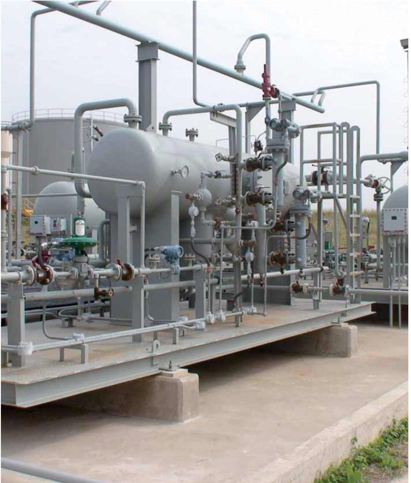
South America: Gas condensate separation plant
